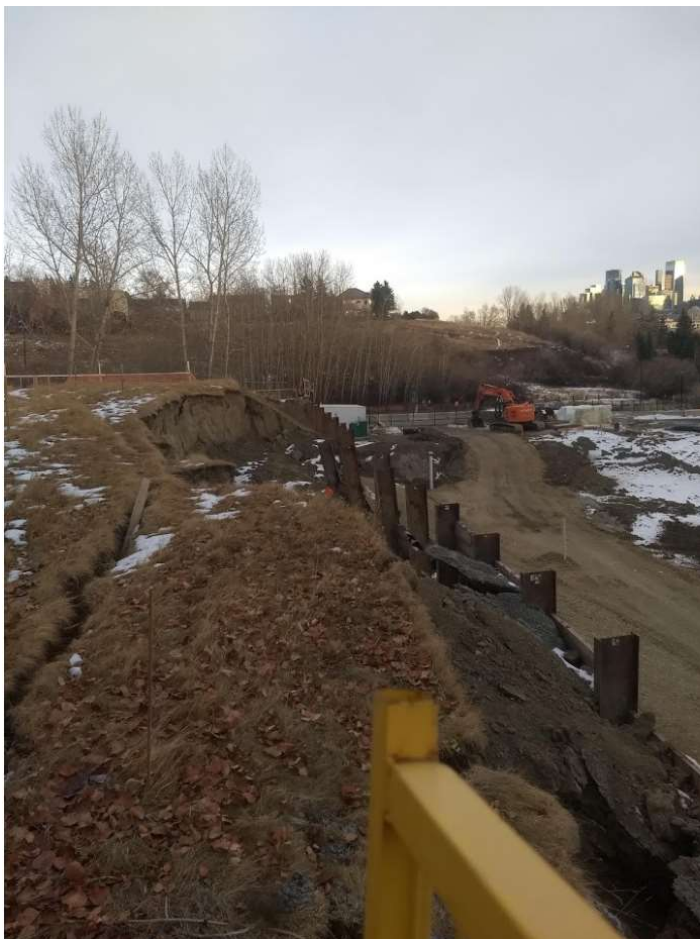
Figure 5 Looking east at the AADAC Adolescent Program construction site. Rotation slumping has resulted in the north wall of the pit collapsing. In doing so it deformed the wood and steel retaining wall constructed to prevent this happening.
