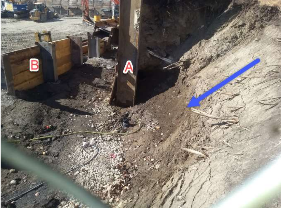
Figure 6 Looking west at the AADAC Adolescent Program construction site. This March 2021 photograph showing (A) the first retaining wall from September 2020 and (B) the second retaining wall from March 2021 built to replace the first set of retaining wall piles. Blue arrow shows angle of repose of the sediments which is approaching a 90% gradient when the soil is dry.
