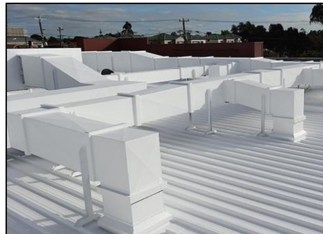
Camouflaging of rooftop equipment by painting the venting with a colour that is harmonious with the roof.
