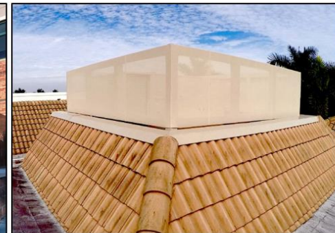
Screening of rooftop equipment with coloured awning fabric that is consistent with the building form and finish.
