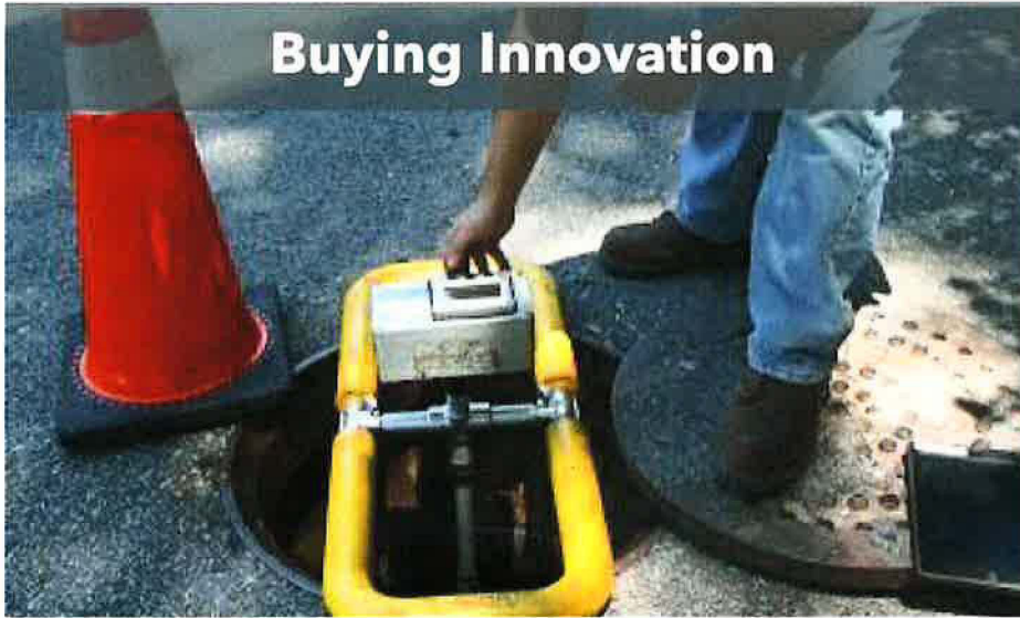
Piloting New Technologies – Sewer Line Rapid Assessment Tool
