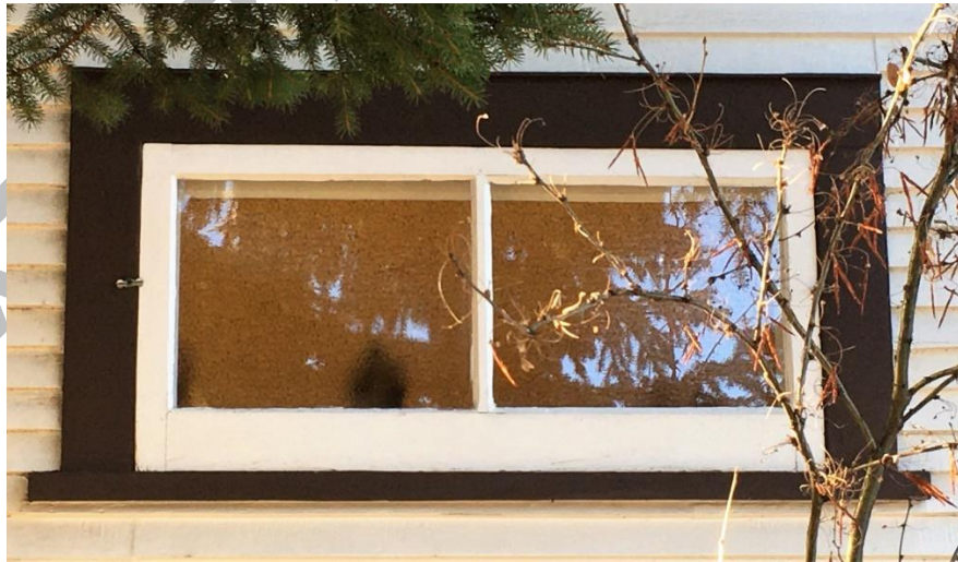
(Image 2.16: Example of fixed one-light wood window with 2-light wood storm window)
