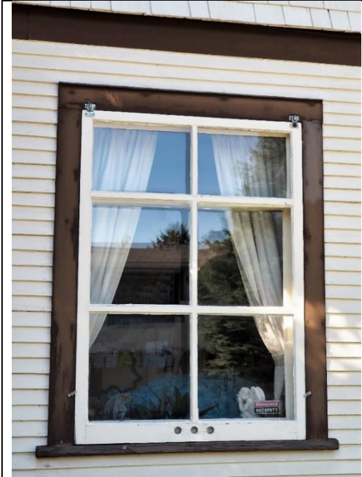
Image 2.11: Example of 1-over-1 single hung wood window and 6-light wood storm window
