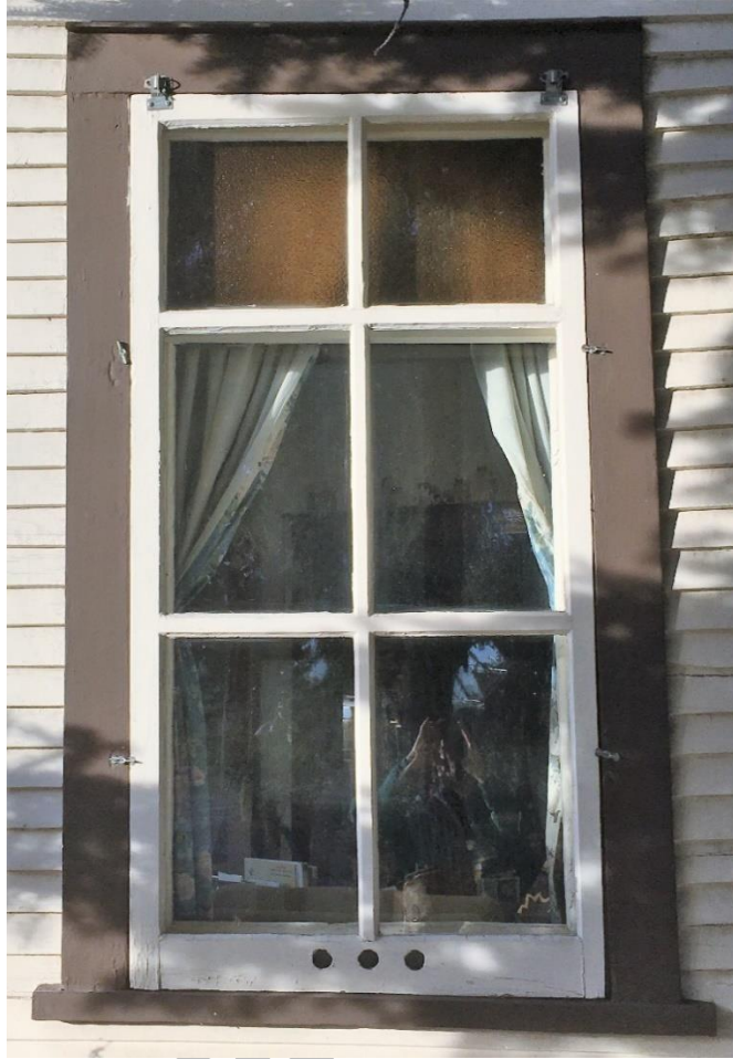
(Image 2.15: Example of 1-over-1 single hung wood window and 6-light wood storm window)
