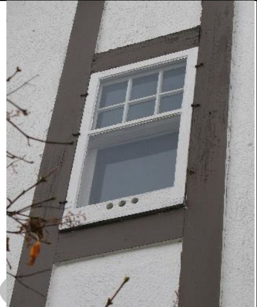
(Image 2.5: example of one of three 6-over-1 wood hung windows with flat heads and painted wood trim)
