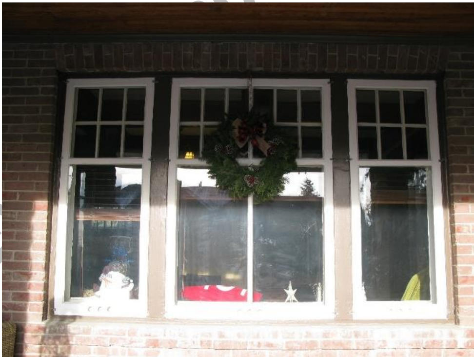
(Image 1.5: triple assembly consisting of a 12-over-1 flanked by 6-over-1 wood windows with sill and flat gauge lintel in concrete brick)
