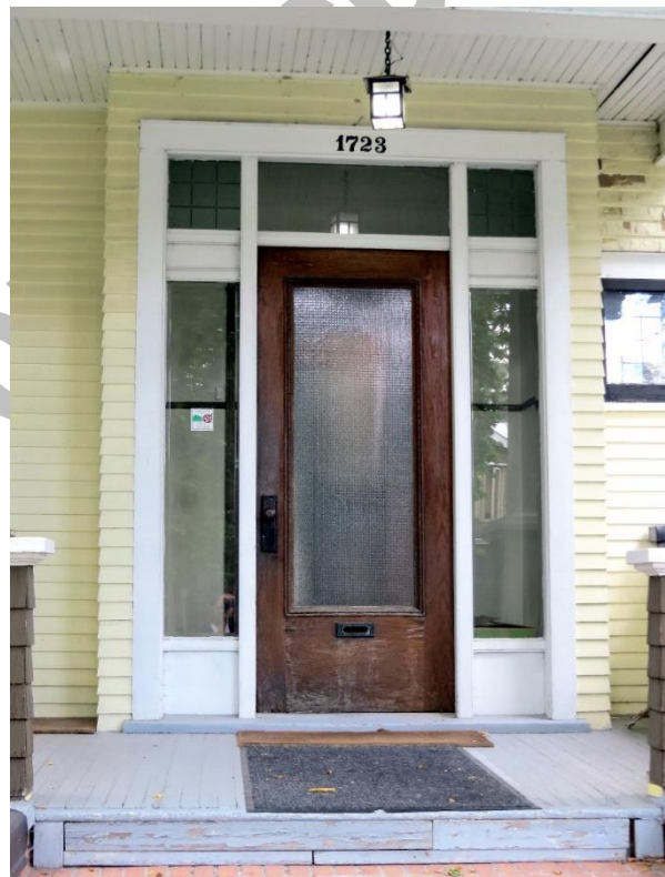
(Image 2.4: Detail of offset front entry on front veranda with side-lights, 3-light transom, wood surround, and original wood door with glazed panel and wood tongue-and-groove ceiling)
