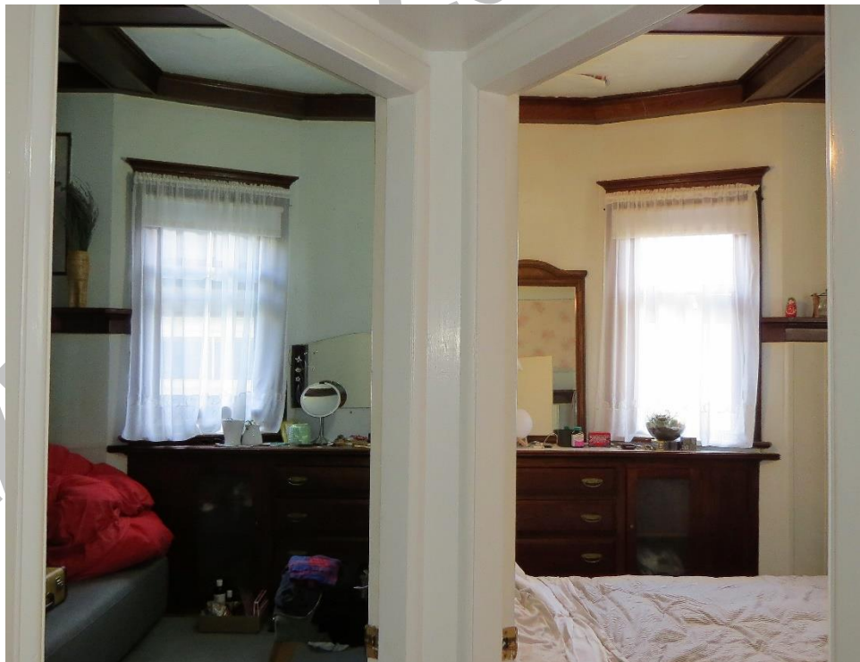
(Image 3.8: Built-in drawers and cabinet (partitioning wall constructed over built-in drawer and cabinet unit during previous renovation))
