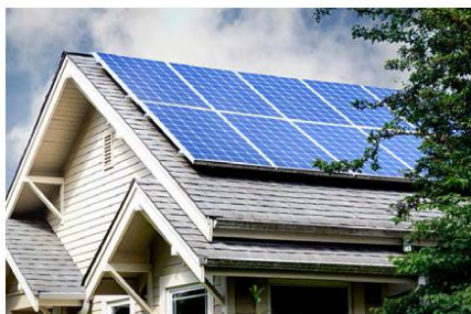
Photo: Solar panels to capture solar energy.
