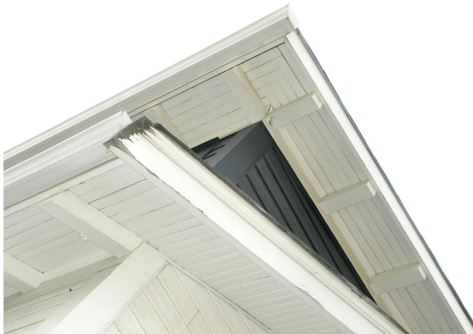
(Image 2.9: detail of typical wood eaves with exposed wood rafter tails with squared (shed roof extensions) or beveled ends (gabled roof); plain wood fascia; wood tongue-and-groove soffits)
