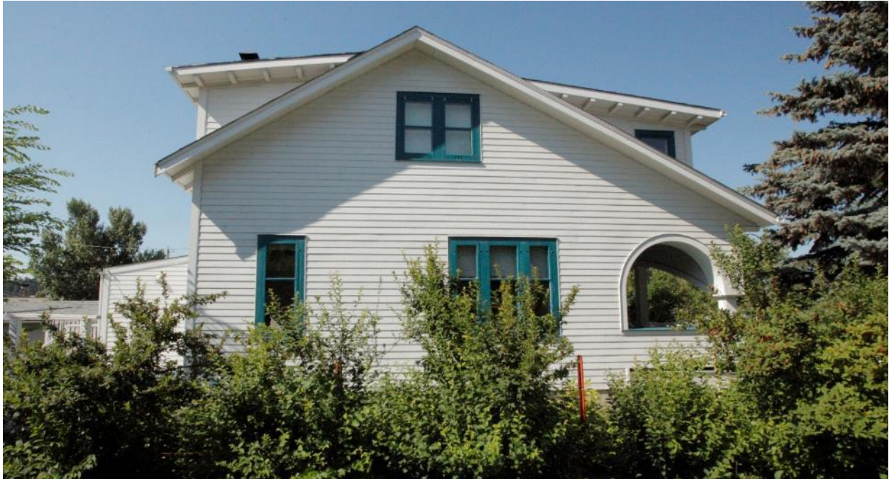
(Image 2.6: Northeast façade showing six 1-over-1 wood windows, three of which are in a triple assembly and two in a double assembly; curved opening on side of porch)
