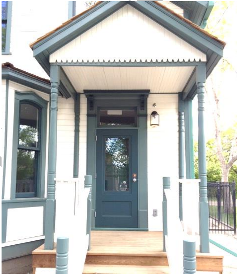
(Image 1.3: Porch and front door surround with decorative crown over single-paned transom)
