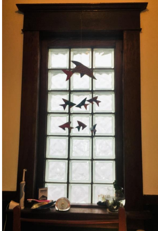
(Image 3.3: Window frame in bathroom)
