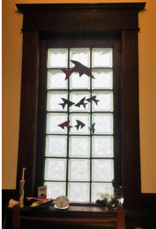
(Image 3.3: Window frame in bathroom)
