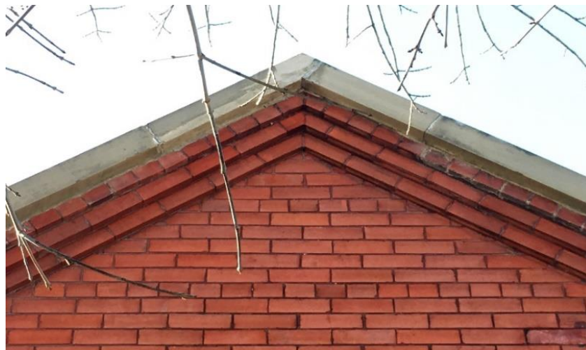
(Image 1.3: Detail of common bond pattern red brick with red-pigmented mortar and corbelled cornice at gable edge with sandstone cap)
