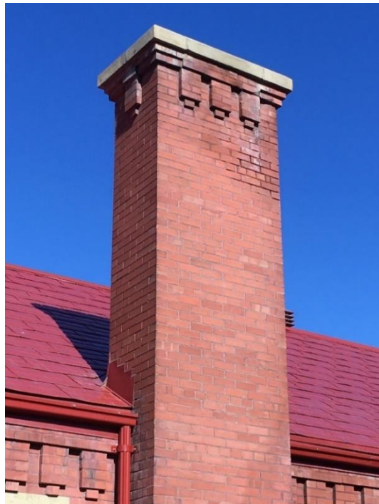
(Image 2.4: Detail of corbelled modillions and sandstone cap of red-brick chimney on east façade of rear addition)
