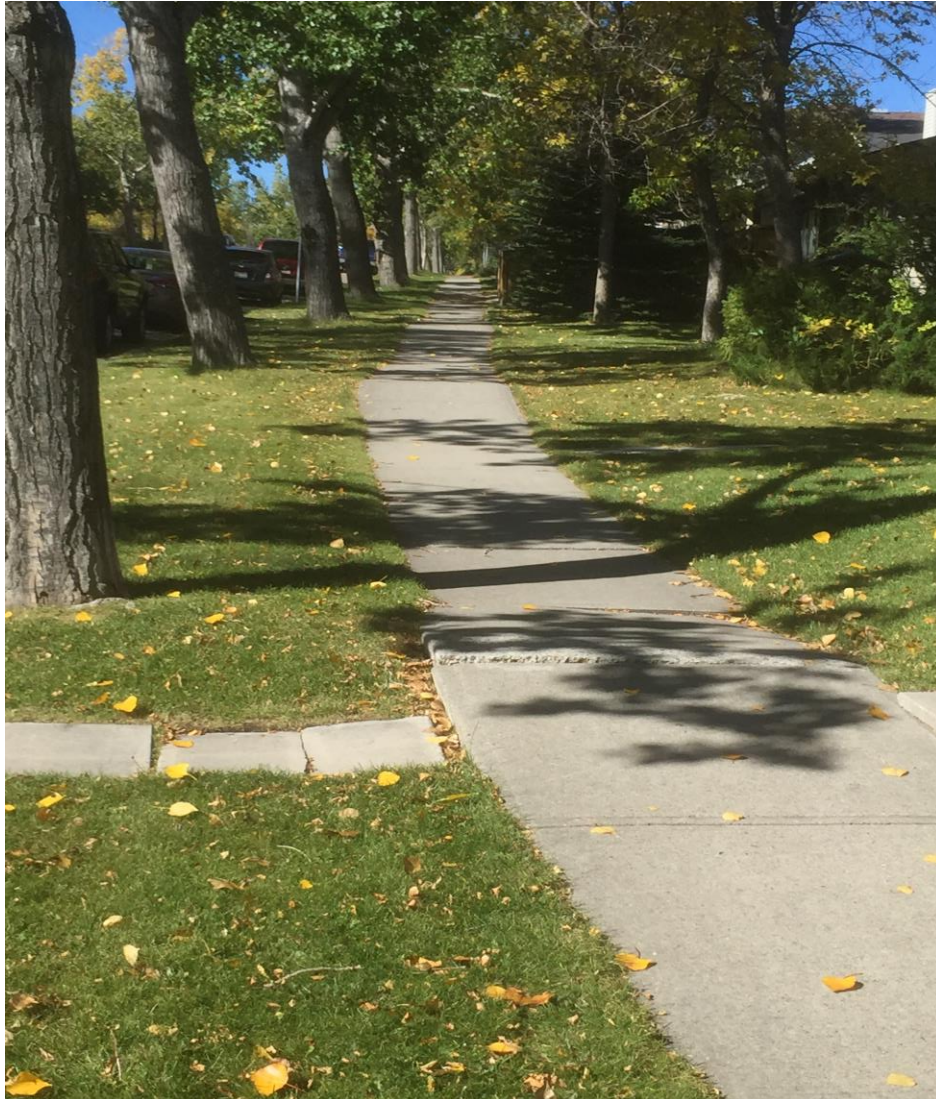
Figure 10: Photo Showing Multiple Tree Root Issues Within One Block Face
