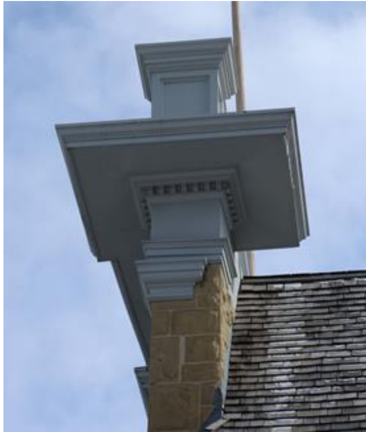
(Image 1.4: Detail of pressed metal entablature as it wraps around 'boomtown' façade)
