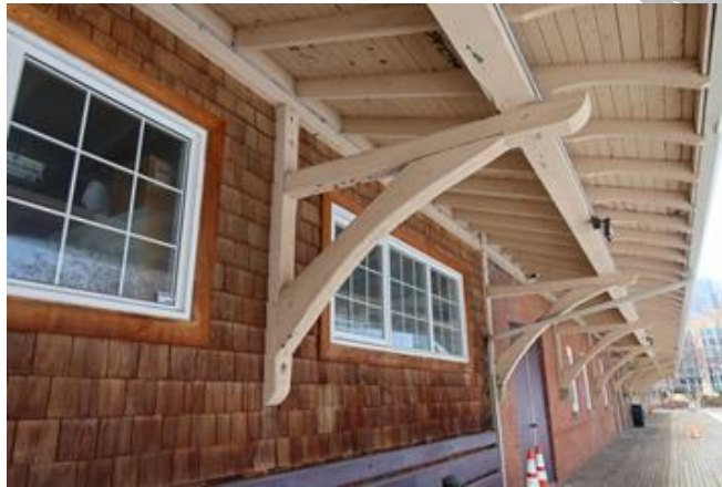
(Image 5.1: Detail of deep eaves with exposed rafter tails and wood soffits, supported by rounded brackets, continuous along east and south portions of St. Mary's Parish Hall/CNR Station phases)
