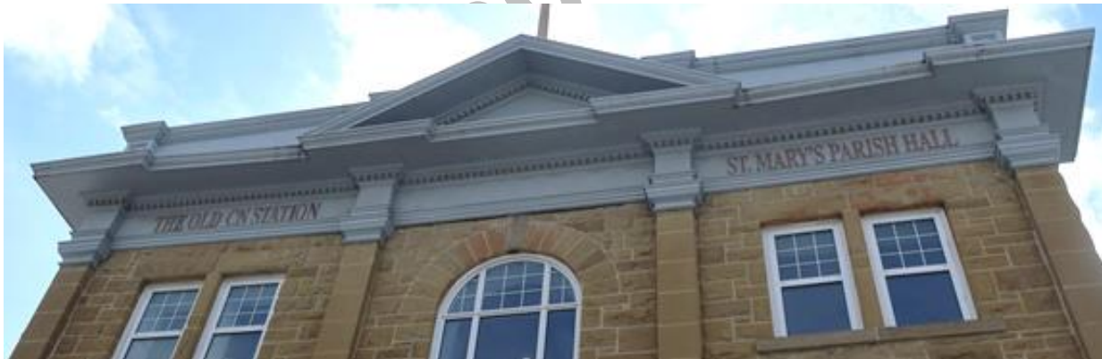
(Image 1.3: Detail of pressed metal entablature with central pediment, string course, voussoirs, rough-faced sandstone lintels and sills)
