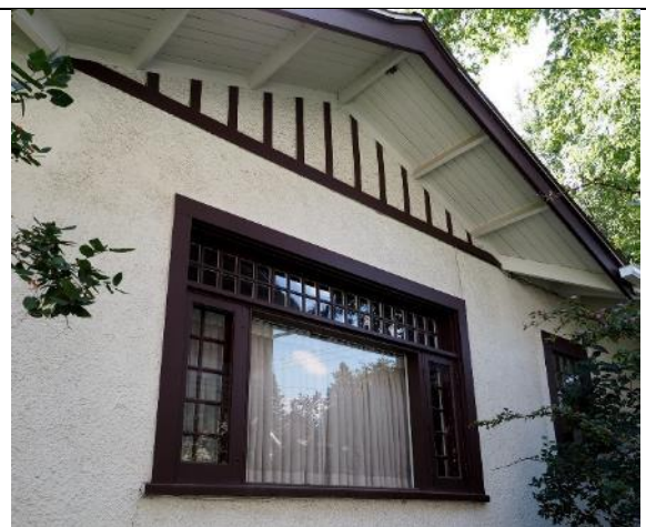
Image 2.3: three-part window comprising side casements with multiple panes (10), multi-pane (36) upper portion and a center fixed-pane.
