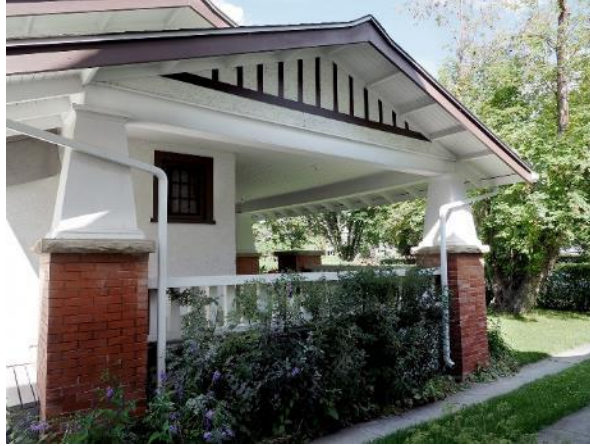
(Image 3.2: south portion of open wrap around porch with with wooden tongue-and-groove ceiling; plain, painted-wood porch balustrade; tapered and paneled columns on brick and sandstone piers)
