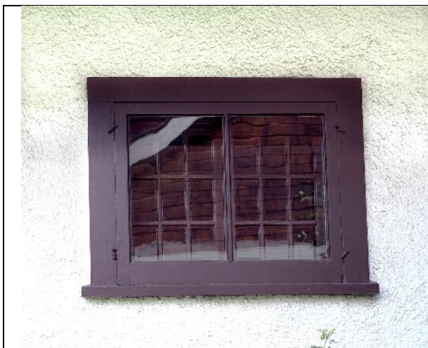
Image 2.2: detail showing one of the two matching windows flanking the fireplace chimney, comprised of two casement windows with multiple panes (9 each)
