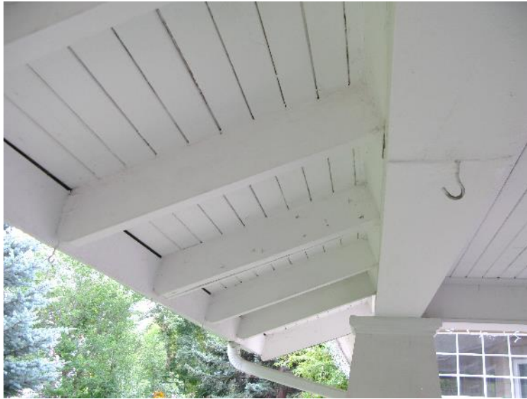
(Image 5.1: example of deep eaves with tongue-and-groove soffits with exposed rounded-end rafters on east roof of wrap around porch)
