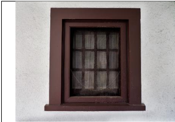
Image 3.3: detail showing one of the two matching casement windows with multiple panes (12 each)
