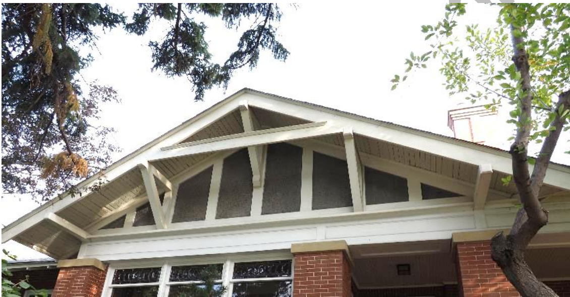
(Image 5.1: Detail of the north gable end; example of the tongue and groove soffits)
