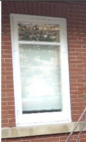
Image 4.5: One of the two most northerly windows with decorative beveled glass transom
