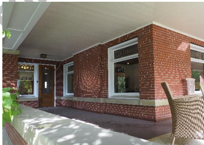
(Image 3.2: View looking northwest at the open wrap around porch with with wooden tongue-and-groove ceiling; continuous sandstone band; side entrance)
