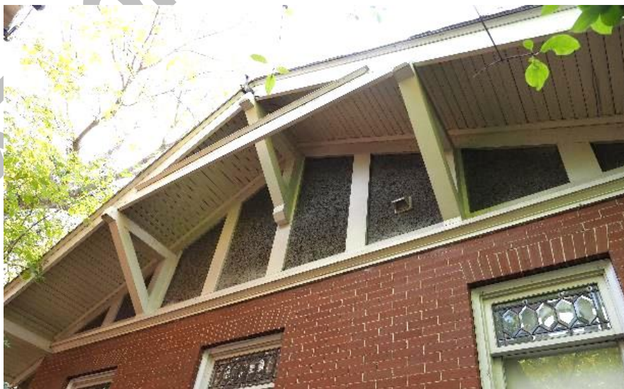
(Image 5.2: Detail of the north gable end; example of the tongue and groove soffits)
