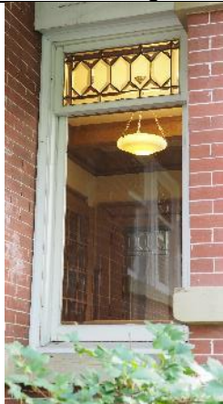
Image 3.5: Hung unit with decorative beveled glass transom, positioned on the east side of the gabled extension
