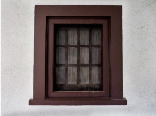
Image 3.3: detail showing one of the two matching casement windows with multiple panes (12 each)
