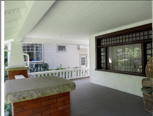
Image 1.3: detail showing open wrap around porch with with wooden tongue-and-groove ceiling; plain, painted-wood porch balustrade; tapered and paneled columns on brick (stretcher-bond) and sandstone piers; brick stairway pedestals with sandstone caps
