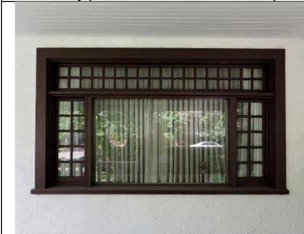
Image 1.5: three-part window comprising side casements with multiple panes (10 each), multi-pane (36) upper portion and a center fixed-pane.
