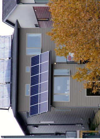
Solar thermal heating and solar photovoltaic panels. Photo credit: David Dodge, GreenEnergyFutures.ca
