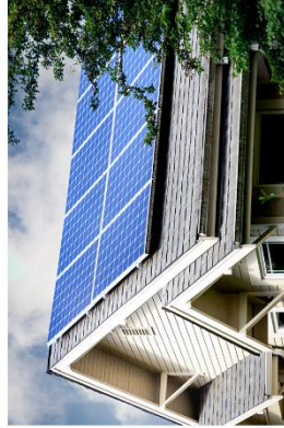
Photo: Solar panels to capture solar energy.
