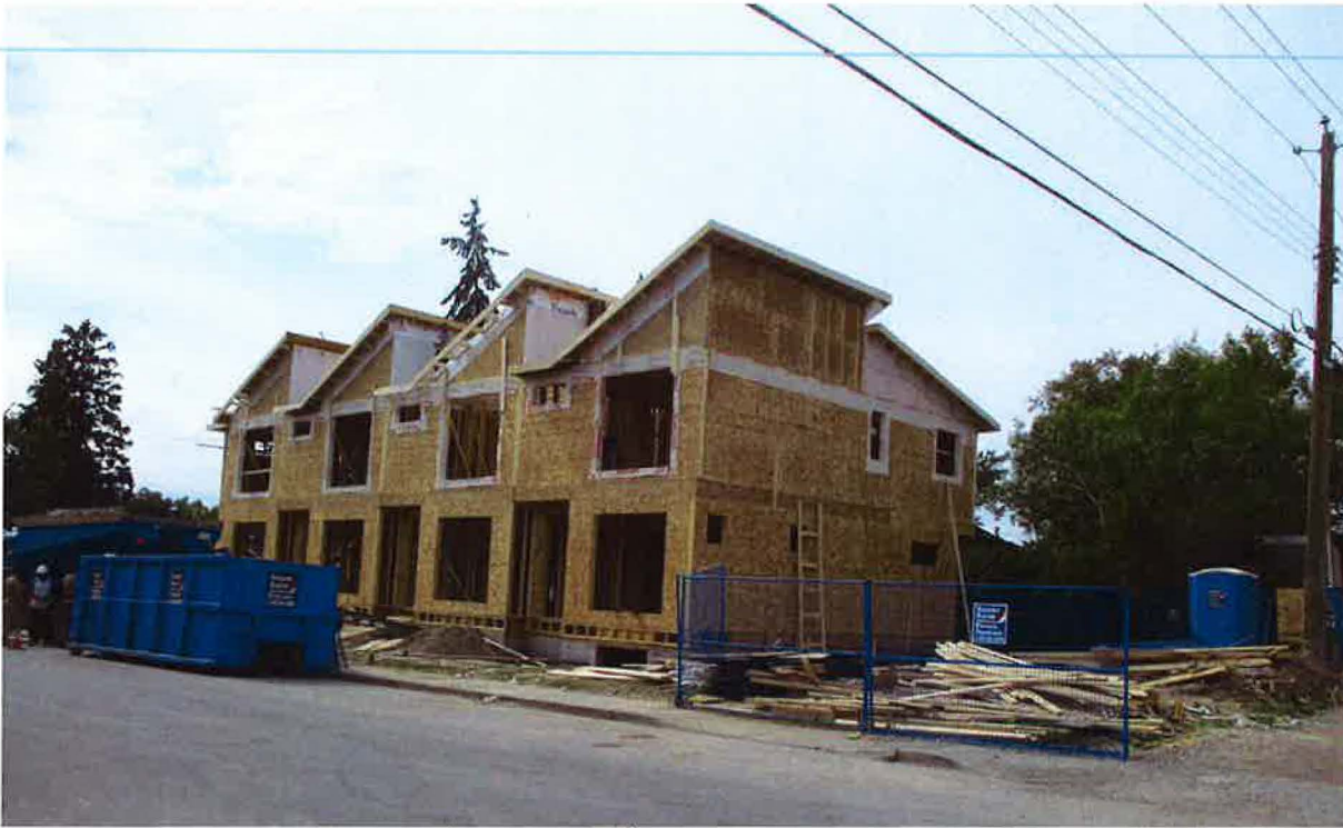
Photo 2: Row housing @ corner of 5 th Street and 20 th Avenue, NW. Note 1. Garages are yet to be built on this property. Note 2: The significant structure to land ratio. Note 3. The structure dwarfs the neighbouring home and overwhelms the neighbour's garden (even without the garages).
