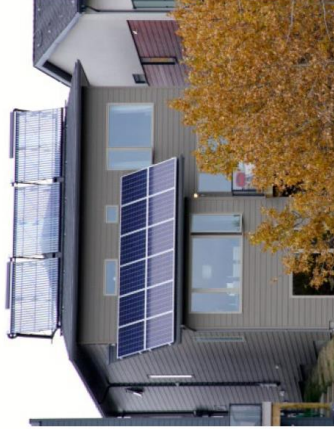
Solar thermal heating and solar photovoltaic panels. Photo credit: David Dodge, GreenEnergyFutures.ca
