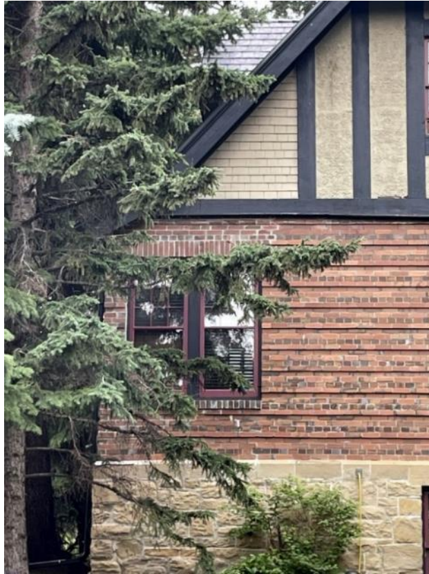
(Image 3.2: Portion of east façade showing typical random ashlar, cut sandstone foundation, banded brick cladding (1 st storey) and decorative wood half-timbering and shingles (2 nd storey).
