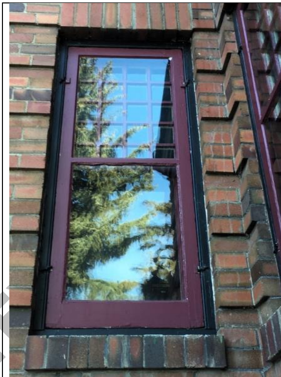
Image 3.7: Example of original fenestration with multi-light-over-single pane wood window with soldier course brick header and rowlock brick sill. Note: Storm window is not regulated.
