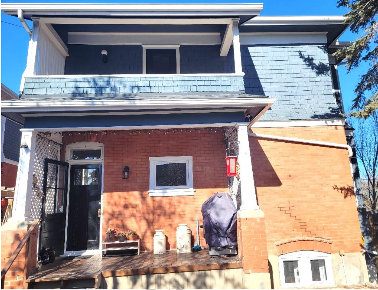
(Image 2.4: South façade – main floor window is not regulated)
