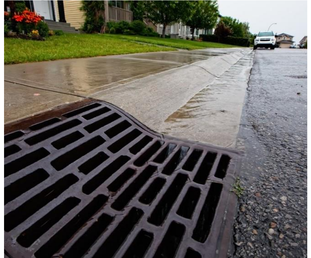
Example of a stormwater grate
